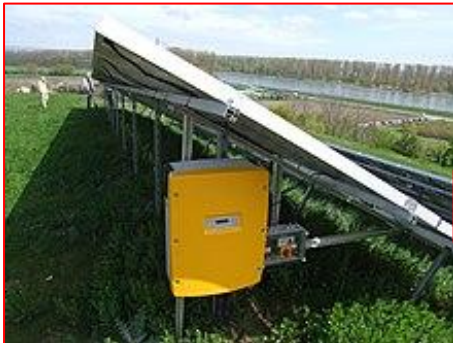
Solar panel with Inverter
